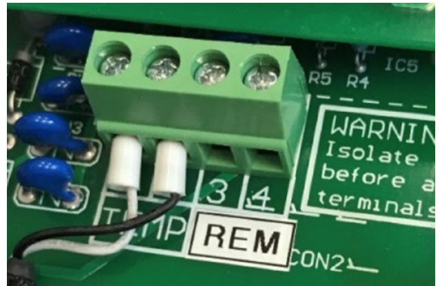
Figure 22: Storage tank terminals 1&2 on block 2 (CON2).
